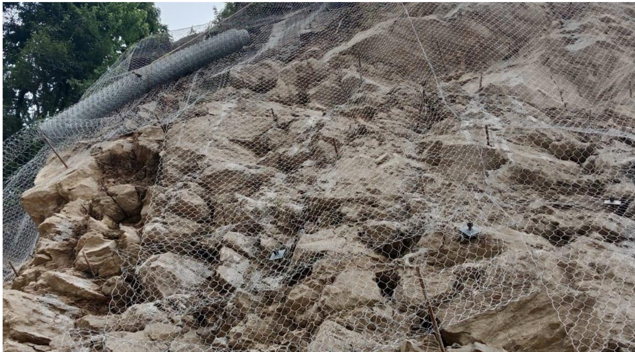
Rockfall Netting on NH-717A, West Bengal
